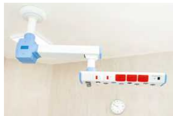
Side view with electrical outlets
